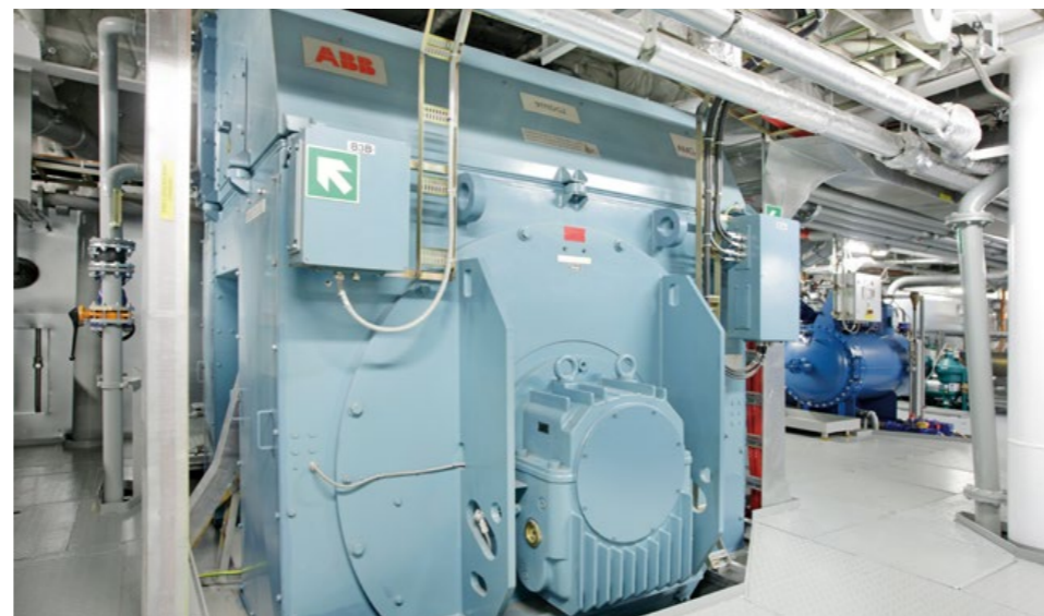
High voltage marine generator
