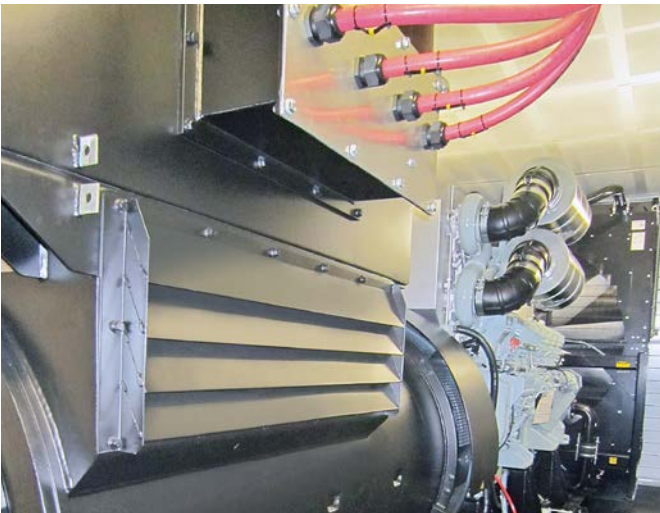
Emergency generator set supplying 2,000 kVA / 11 kV
