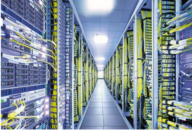
Demanding data center application
